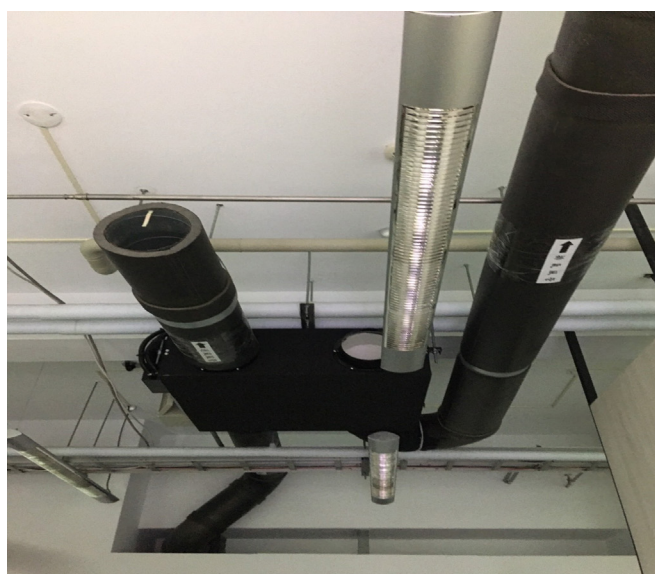
Figure 1: Test laboratory (from left to right in the image: main experiment area, central cabinet, and office area, equipped with two FCUs and one energy recovery ventilator at the top).
