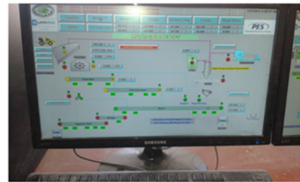
Figure 5: Crusher operator station.
