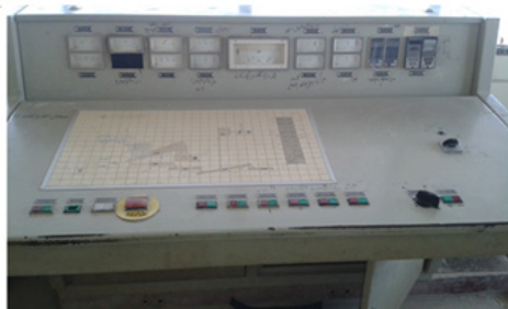
Figure 4: Old control and operation system.
